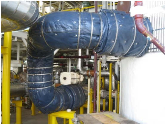
J30 jacketing on pipework and flanges, CPOC Platform
