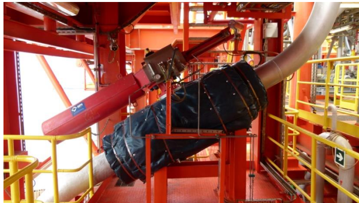
J90 Ball valve jacketing on the Teekay FPSO
